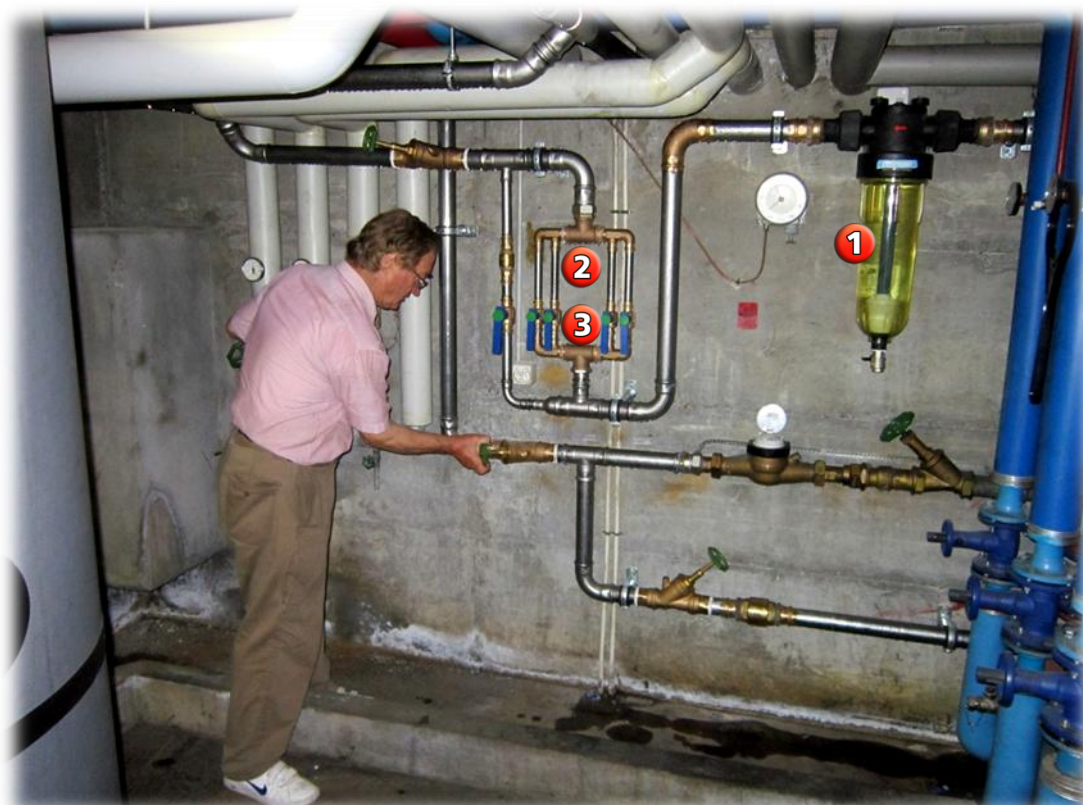
Installation for a building of 35 housing
